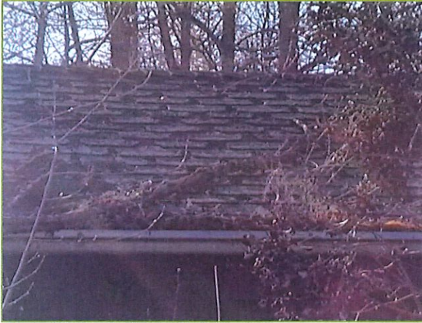
Figure 22. Roof with debris buildup
